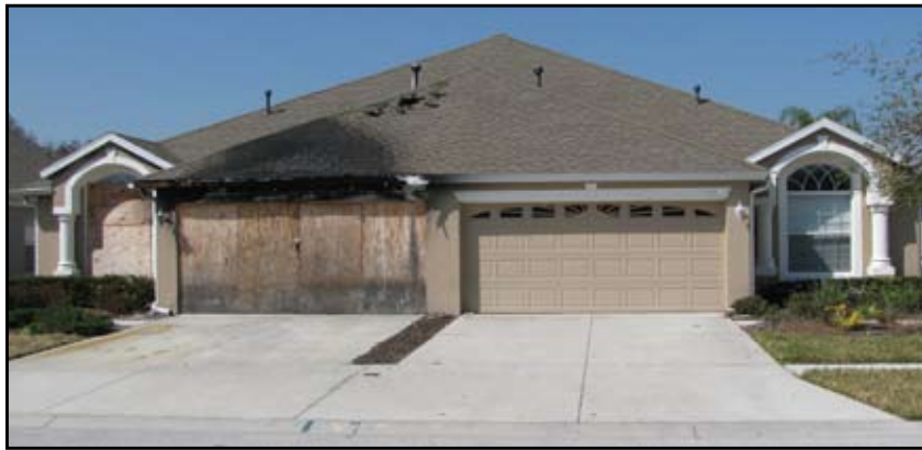
Damage from a fire in the boarded-up villa at left has rendered its partner at right uninhabitable for more than one year.
